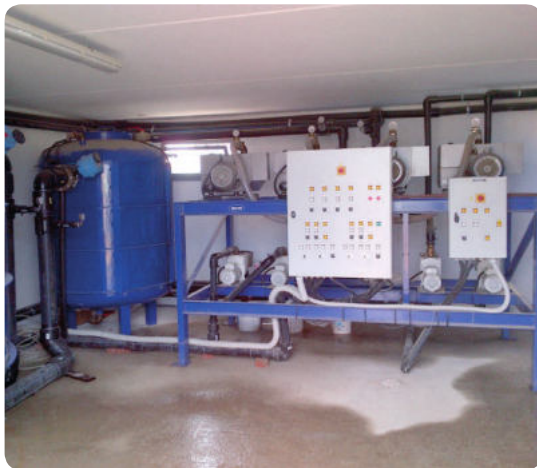
Sewage and Bilge water Continuous vacuum pump out and treatment station.
